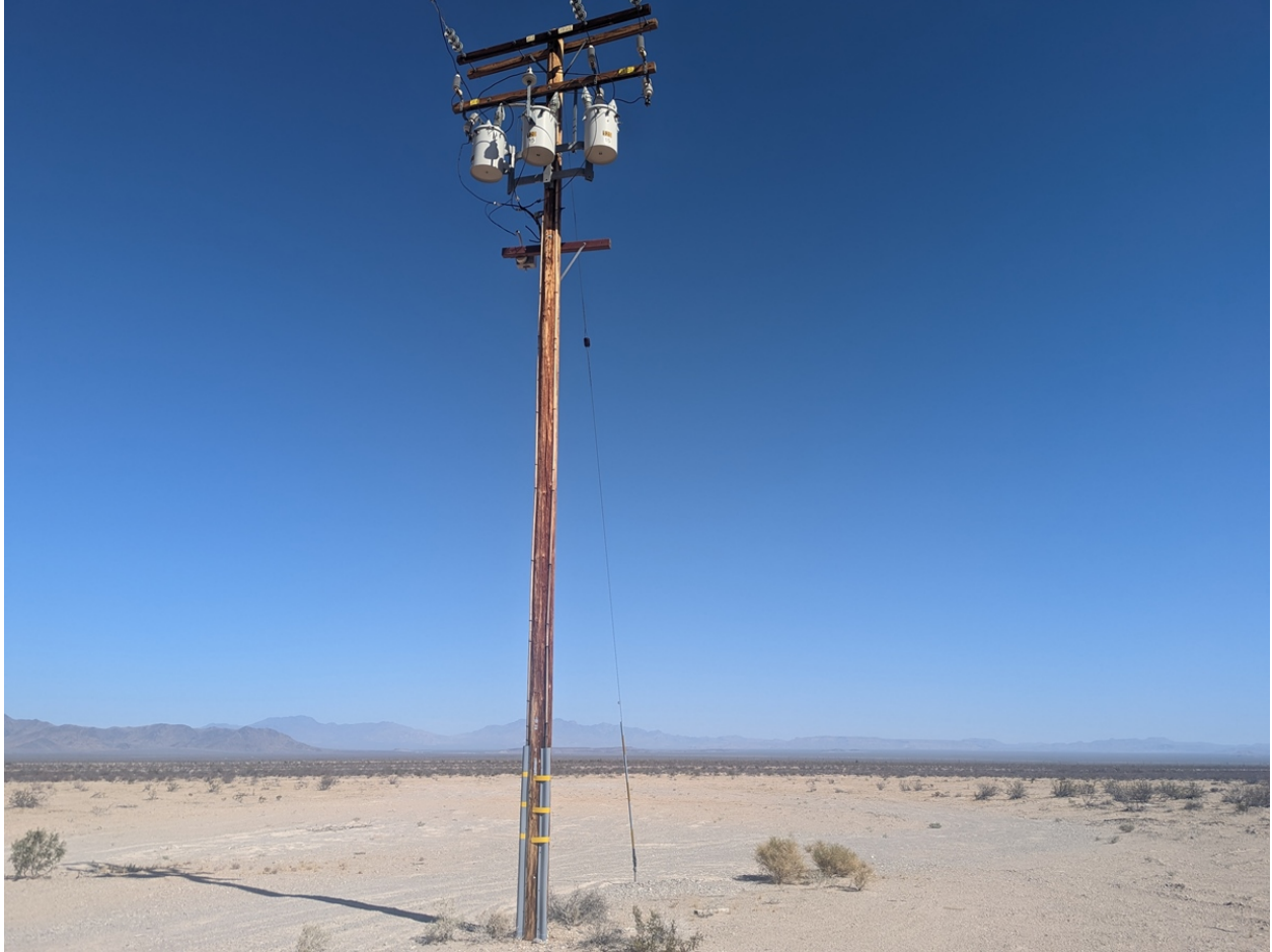
Figure 7: A utility pole
